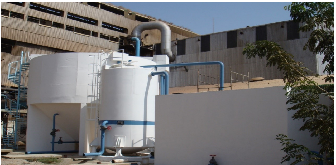
Sedimentation tank, pressure filter, storage tank at Asalaya Sugar CO. Water Treatment
