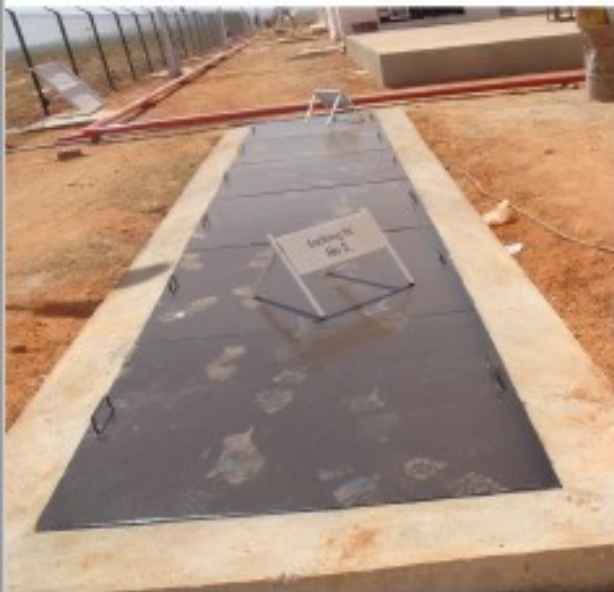
Earthing Collection Manhole
