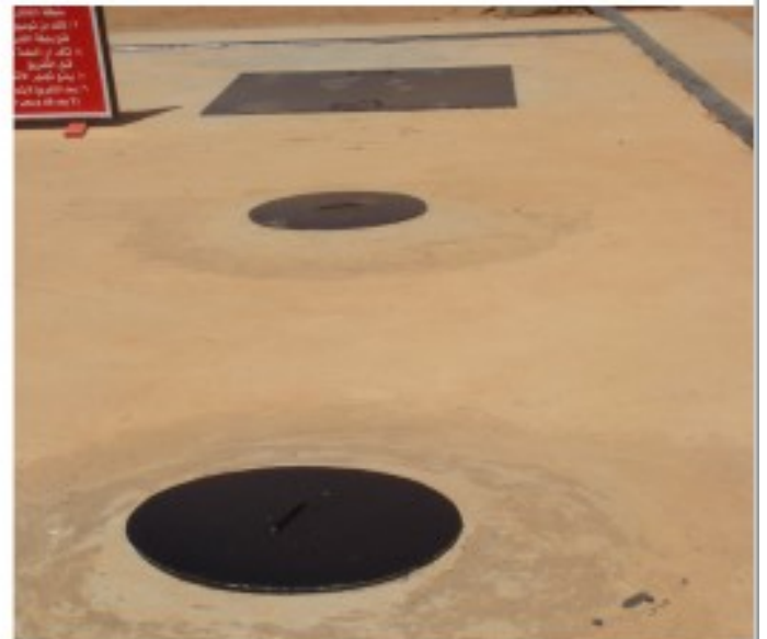
Under ground Tank R.C cover
